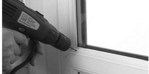
5. With the drill at 90° to the surface, drill Ø2.5mm hole 1 off on each side.
